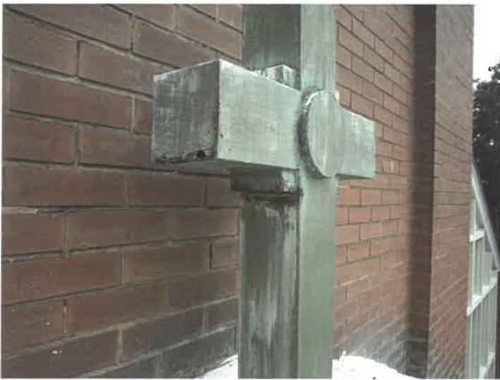
Rusted through and corrosion on the cross, front of church
