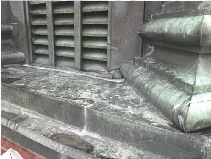
Sheet metal layers exposed over the years, needs caulk, sealer to weatherproof
