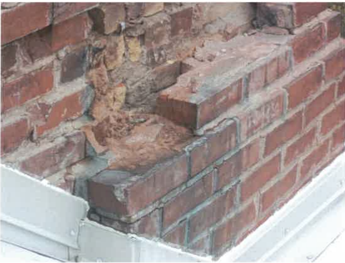
Inside layer, brick deterioration
