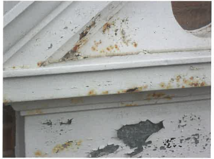
White sheet metal, to repair & repaint
