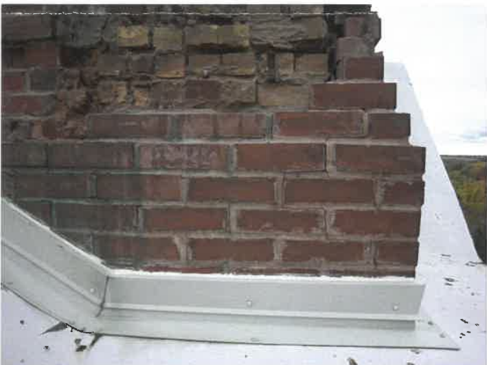
Brick repair: You can clearly see hairline cracks in the masonry, and the backup wall is wet – moisture infiltration
