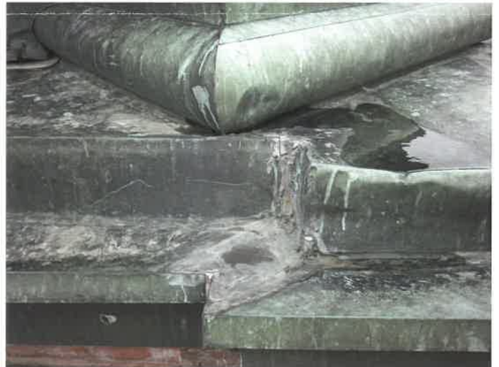
Standing water, showing the cap is not properly shedding water, leads to future corrosion & leaks
