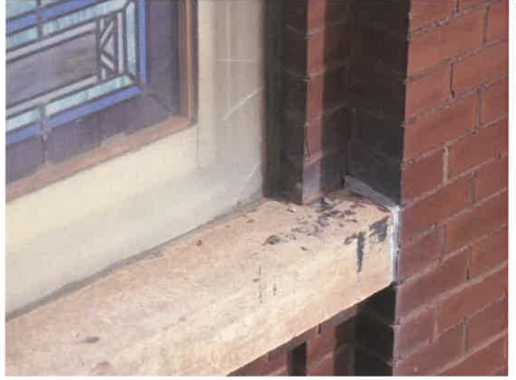
Caulking at stone head joints should be cut out & replaced
