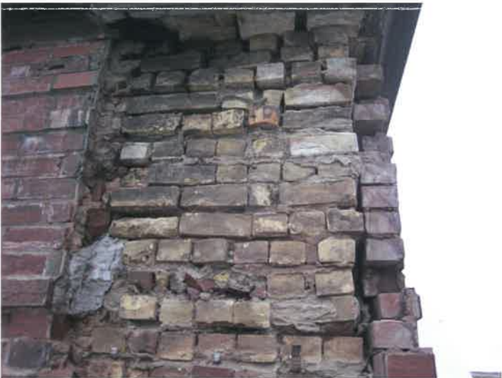
Moisture has been getting into the backup bricks for years, leading to premature deterioration of exterior face brick
