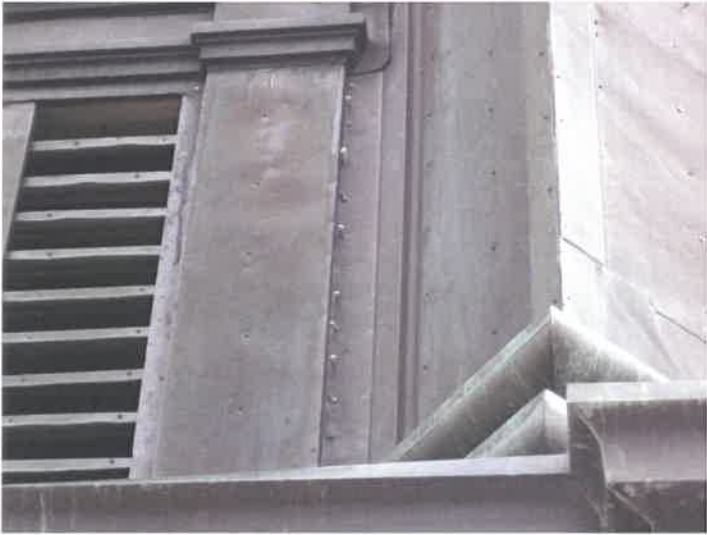
Loose or rusted sheet metal screws to be replaced on steeple
