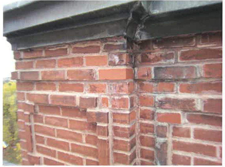
Some mortar joints to be cut out and then bad brick replaced
