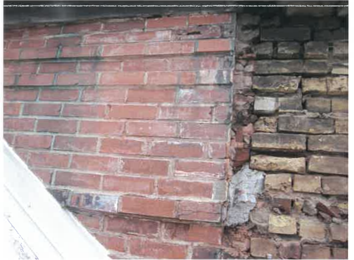
A lot of brick taken from this area were either hand pulled out or crumbled when cutting mortar joints
